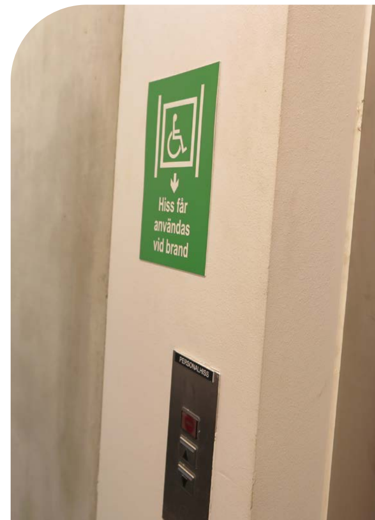
Image 24 | Evacuation lift sign at Sweden's Nationalarenan
